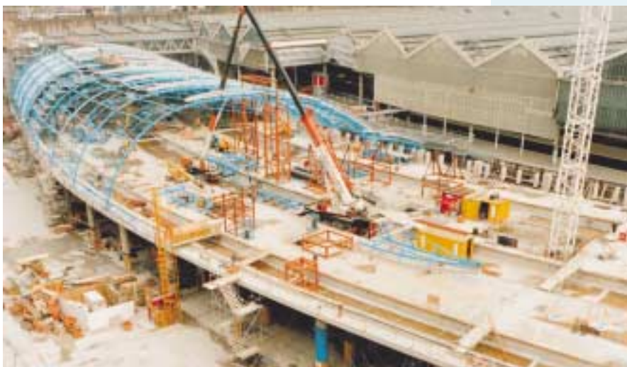
Waterloo International Terminal – Concrete track and platform structure: fast, on time and on budget. (Photo: Lilley Construction)
