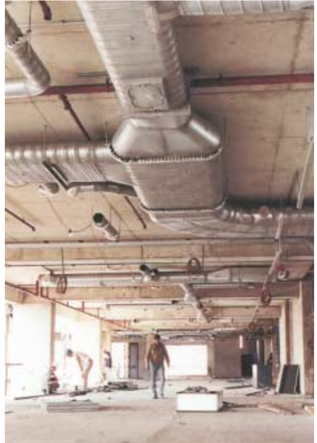
South Quay Plaza, London Docklands – Flat slab construction for freedom to route services.
